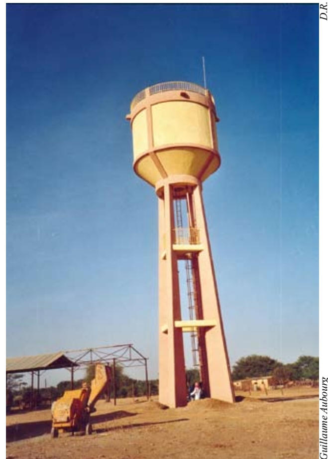
Reservoir for a drinking water supply network in a village in Dioncoulané, Mali
